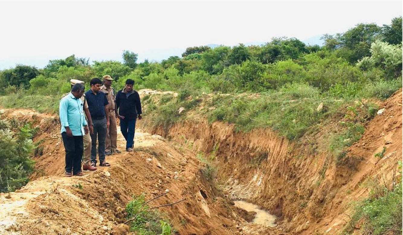
Figure 53: Picture of an Elephant Proof Trench in South India: Image credit: THG publishing Pvt. Ltd.
