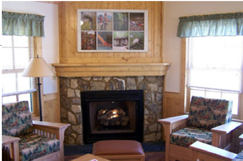
A gas-powered fireplace and fireplace vents
